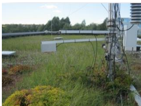
Fig.4. LOG 32 placed on 50 cm above the green roof Source: original
