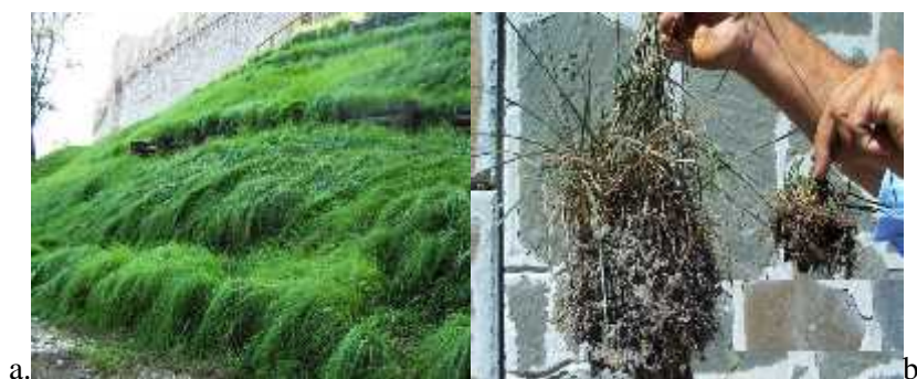
Figure 5. Technology PratiArmati a. consolidation of a slope using technology PratiArmati; b. comparison between technology PratiArmati and traditional plant Source: http://www.pratiarmati.it
