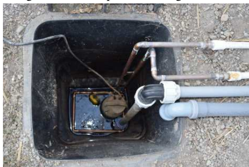
Fig. 3. Tank for the collection and recirculation of the water excess
