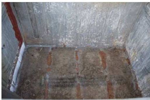
Fig. 5. Tank for composting, internal view
