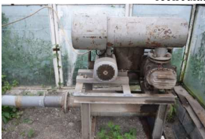
Fig. 4. Compressor for the air flow
