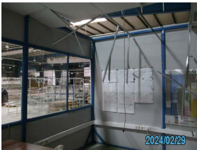
Fig. 5 The damaged NW corner
