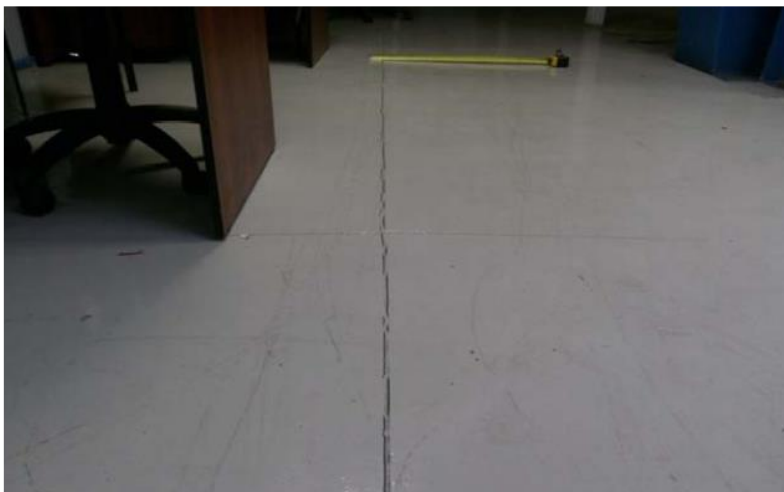
Fig. 6 Crack in the office floor
