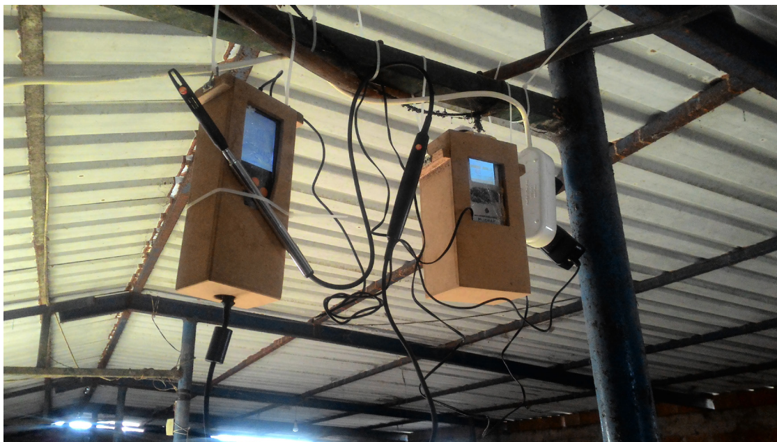
Figure 2. General condition of measuring devices in the shelter
